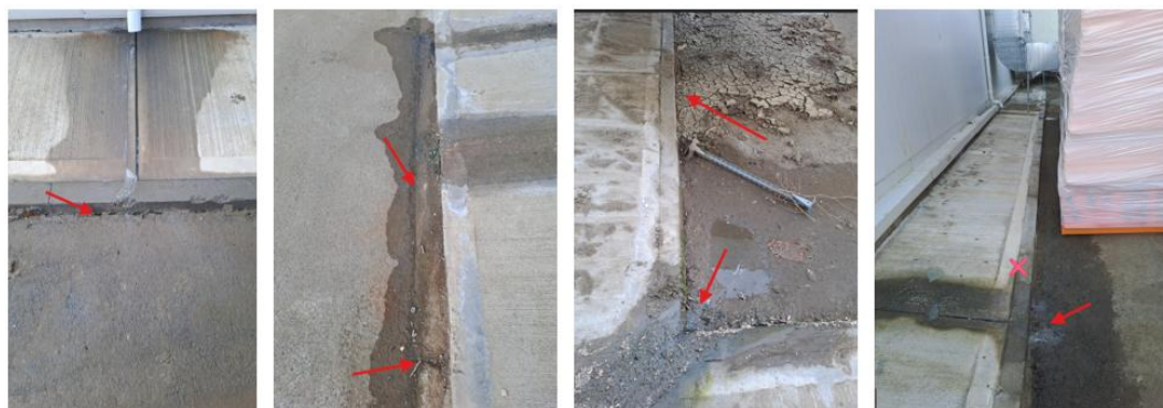
Figure 3 Infiltration of industrial and stormwater
